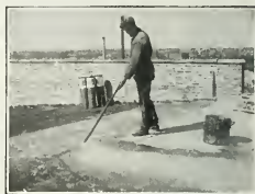
The concrete roof-deck is heavily mopped with a uniform coating of Barrett Specification Pitch.
