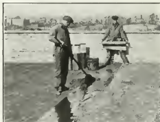
Right: Laying the Barrett Specification Tarr'd Felt on the pitch seal coat. Four plies with pitch in between are laid over the entire roof surface, each ply overlapping three-fourths of the preceding ply.
