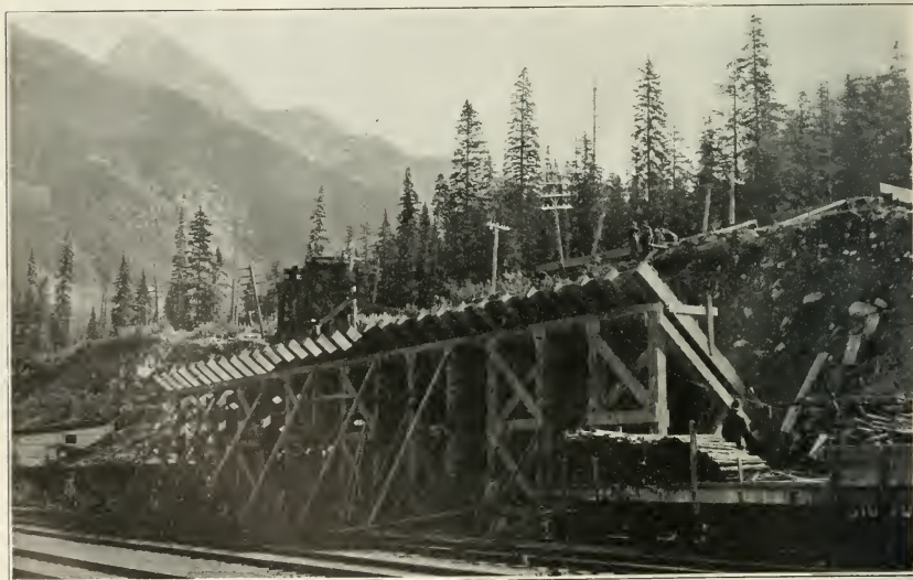
Timber Bunker, for Storing Gravel for Concrete Lining of Connaught Tunnel, C.P.R.
