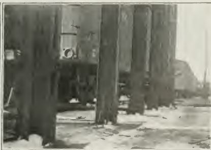
Fig. 1. General view of jacking frame. Fig. 2. Vertical members, screw jacks and height adjusting blocks.
