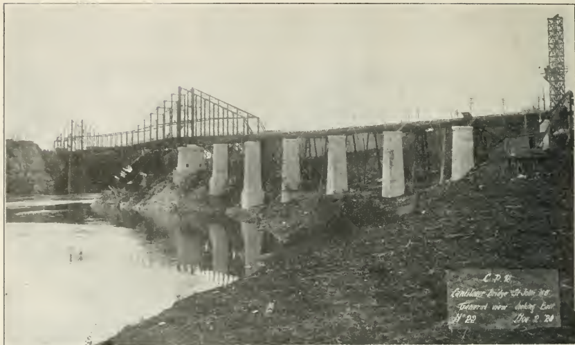
C.P.R. Cantilever Bridge, St. John, N.B. General view, looking east, Nov. 2, 1920. This illustration shows, in the foreground, the substructure of the western approach viaduct to the new bridge.
